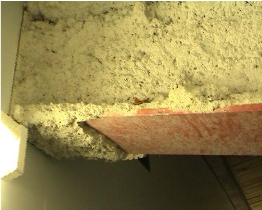
Figure 67 Poorly maintained structural protection of I beam in hallway between suites and players area
