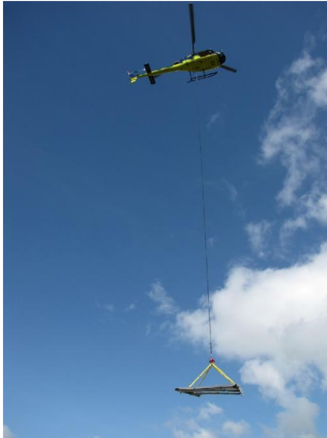
Figure 5: A pre-assembled tower panel is delivered to site for later erection by gin pole
