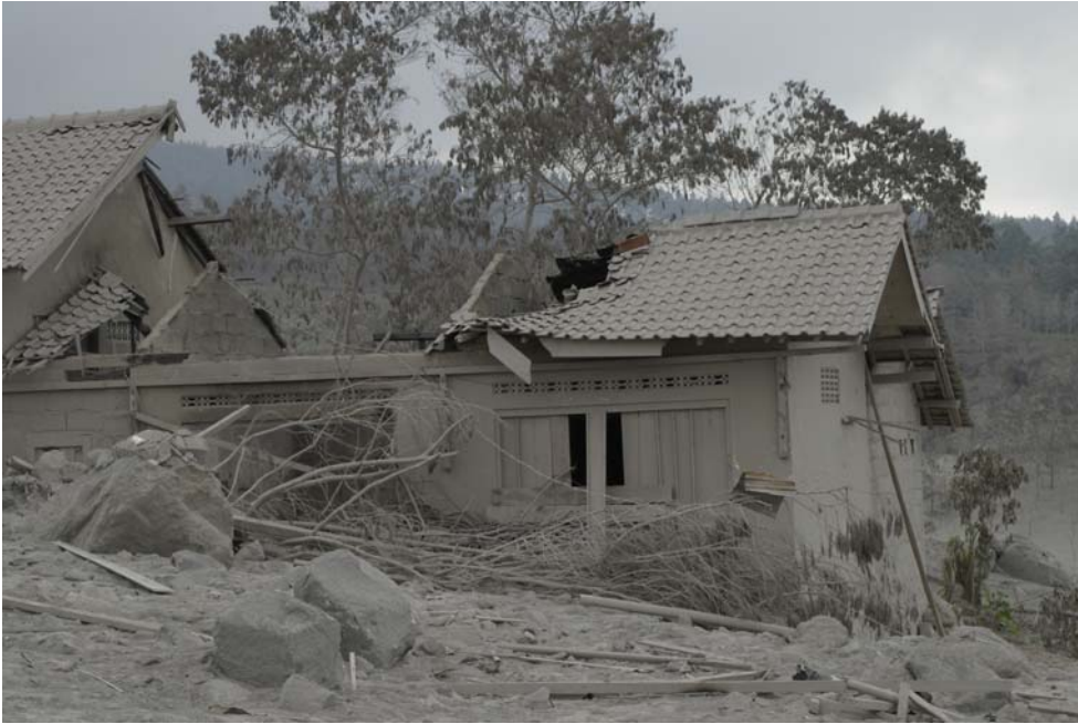
Figure 15 House destroyed by impact of blocks during 14 June 2006 block and ash flows
