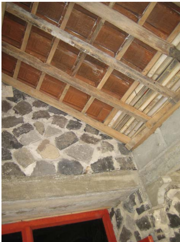
Figure 26 Interior of typical house in Merapi region showing lava block masonry and bamboo and clay tile roof
