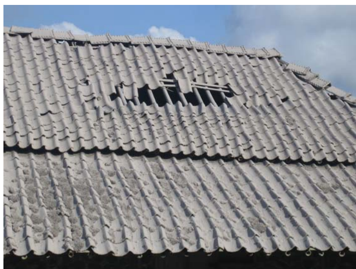
Figure 28 Damaged roof in Petung
