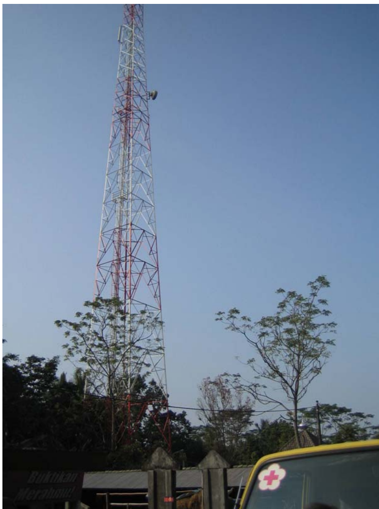
Figure 27 Cellular repeater antenna near Kaliadem
