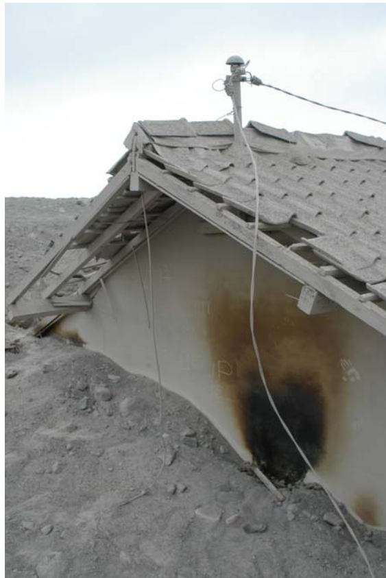
Figure 16 Partially-buried and scorched house in Kaliadem
