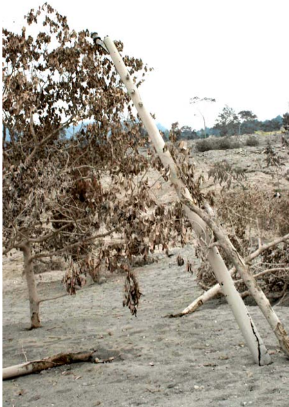
Figure 31 Snapped electricity pole in Kaliadem
