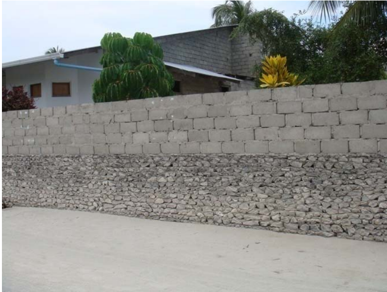
Plate 4-4. Outer wall of house in Dharavandhoo. Cement bricks have been laid over the older coral wall.
