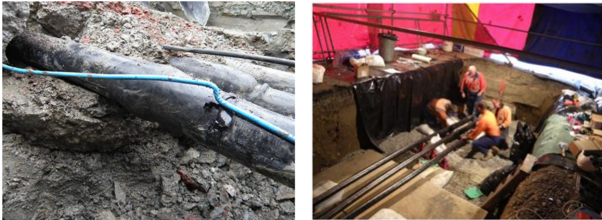
Figure 1. 66 kV underground cable distribution network: a) damage to 1600Cu XLPE cables; b) repair activities (photo credit Orion).
