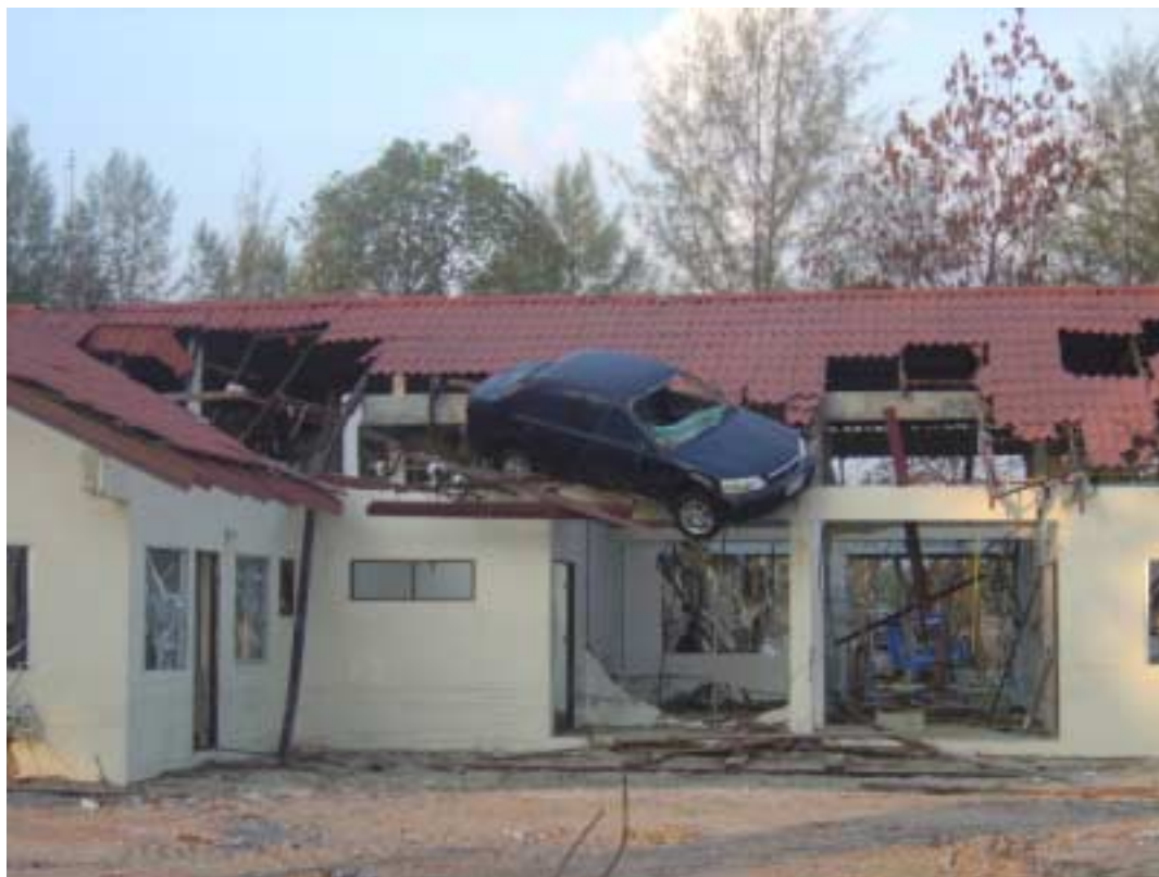
Figure 4. Tsunami wave heights were inferred from strand-lines and watermarks on buildings. In this case a car was lifted above the roofline of a resort in Khao Lak (Photo Thai Meteorological Department).
