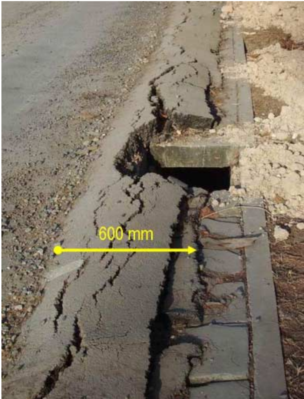
Figure 10. Damage to roads was locally severe due to scouring. At Kamala Beach, Phuket Island, where the torrent depth was 3-4 m, the beach-front road pavement was shifted landward 600 mm onto the adjacent stormwater drain cover.
