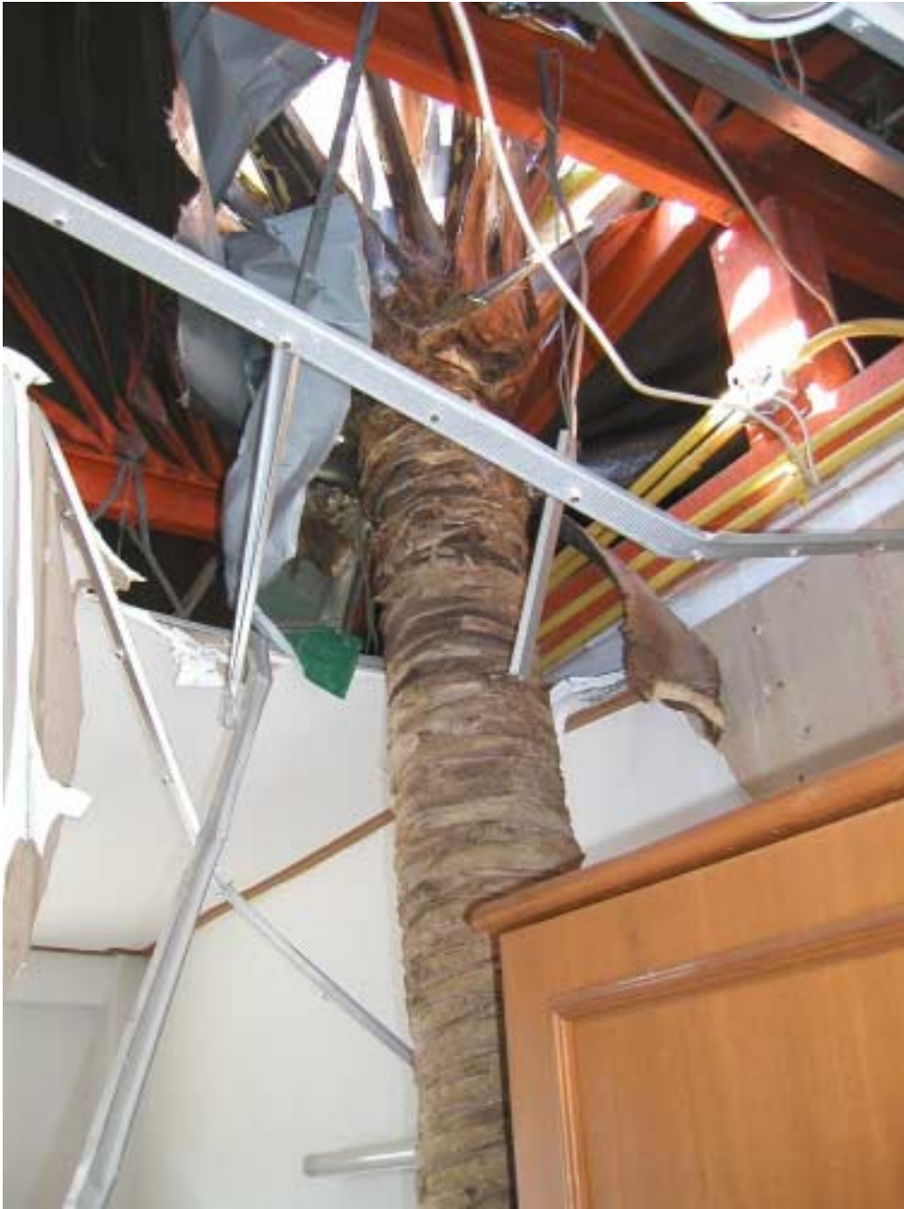
Figure 14. Extraordinary volumes of debris were entrained by the tsunami and contributed to its destructive impact. This coconut palm trunk penetrated the roof and internal ceiling of a hotel on Koh Phi Phi (Photo ED).
