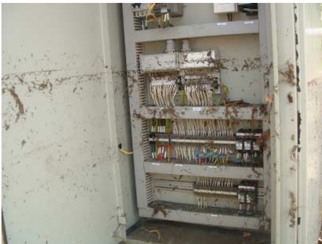
Figure 9a and 9b. Inspecting damage to a sewerage pumping station at Kata Beach, Phuket Island. Electrical control systems were damaged beyond repair, causing sewer overflows into the adjacent stream, and discharge onto the nearby beach (Photos RB and HC).
