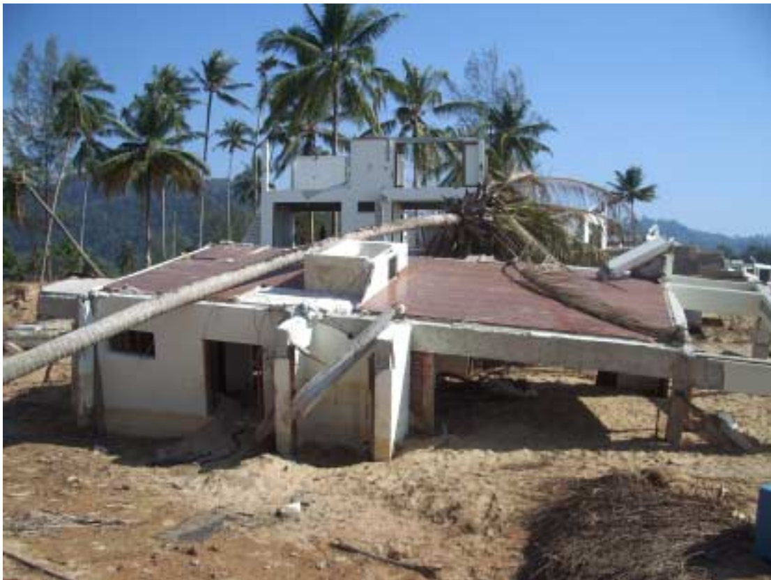
Figure 15a and 15b. The receding waters after each wave caused substantial scouring of small streams and low-lying depressions, as shown here at Khao Lak. The scoured “channel” (15a) is 50 m wide and up to 3 m deep, completely undermining the resort buildings (15b) nearby (Photos RB).
