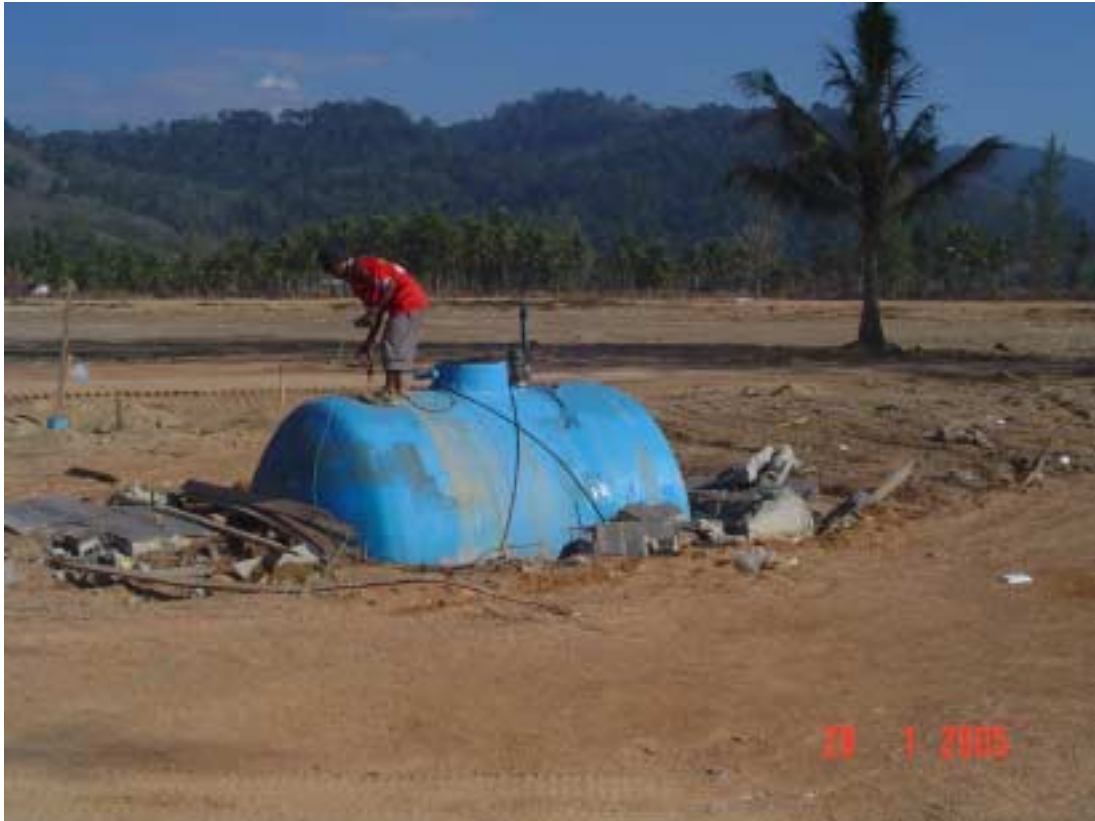
Figure 16. Liquefaction of soils appears to have occurred during the surge and withdrawal of tsunami waters at Khao Lak, with underground services such as this tank floating to the surface (Photo NE).
