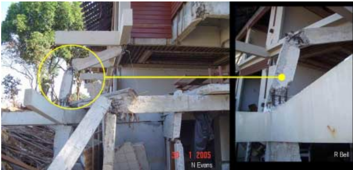
Figure 12. Damage to reinforced concrete frame structures was only locally severe, where exposed structural elements were impacted by entrained debris (Photos NE and RB).
