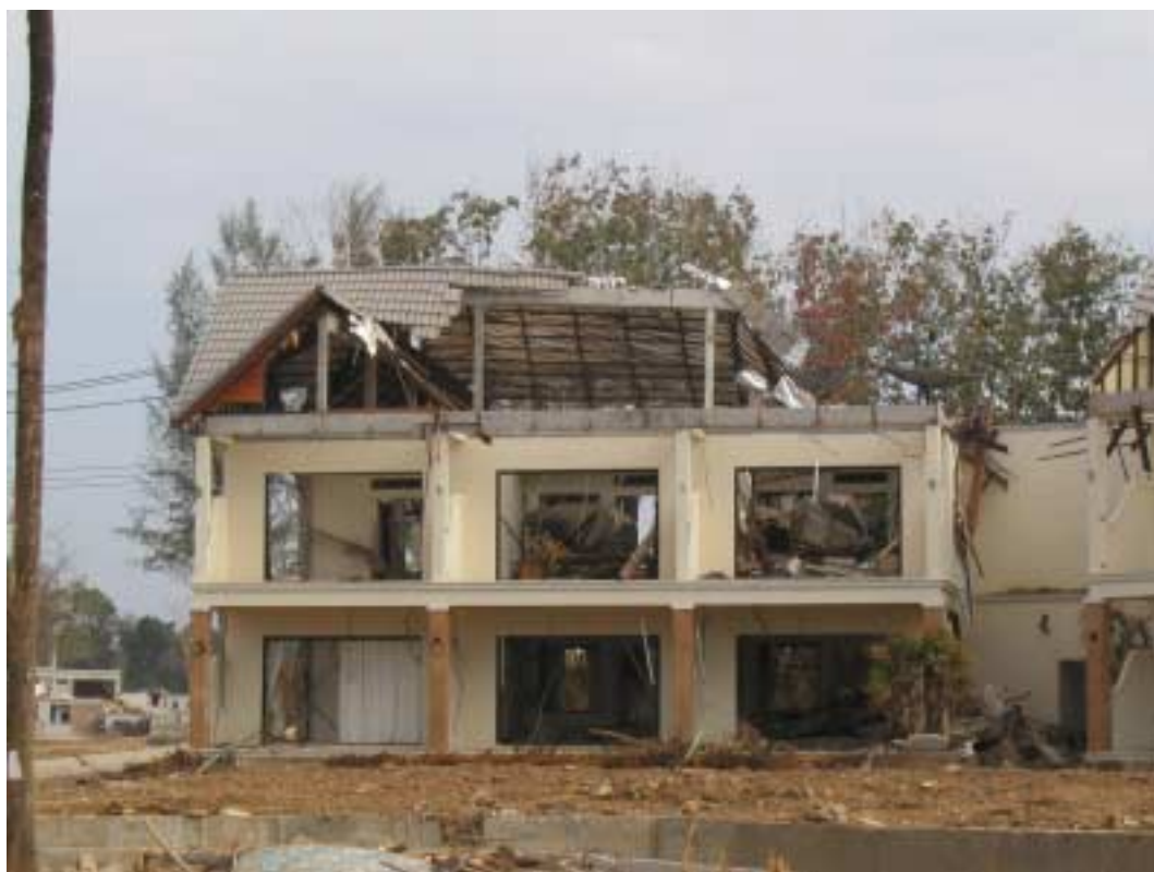
Figure 5. Missing roof tiles indicate the tsunami torrent depth exceeded nine metres at this location in Khao Lak (Photo ED).
