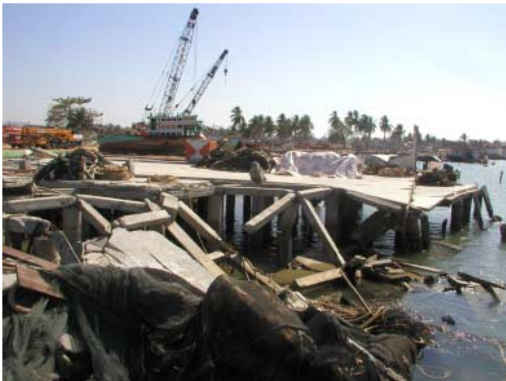
Figure 17. Severe damage to the wharf piles and topping at Ban Nam Kem, a fishing port north of Khao Lak, where the tsunami height reached nine metres (Photo HC).
