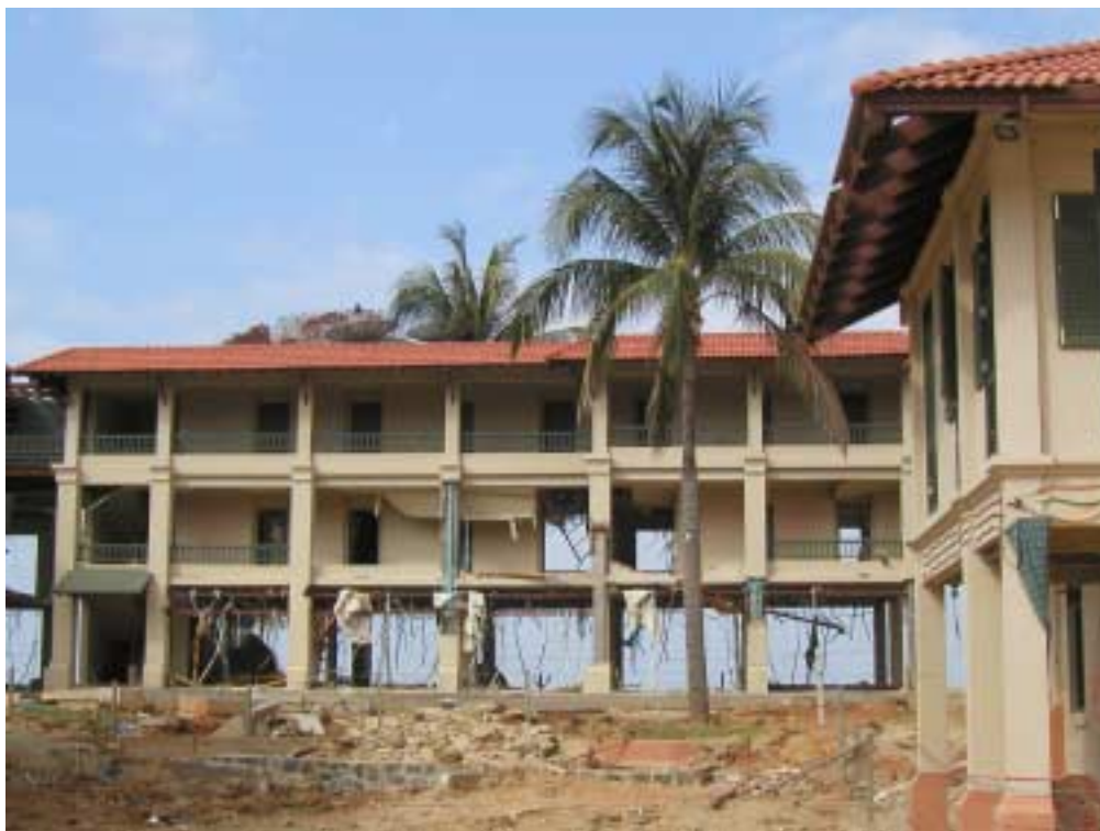
Figure 13. One of resorts at Khao Lak located a few hundred metres from the shoreline, where the highest tsunami run-up (12 m) occurred. Water entered rooms even on the third floor, and in-fill block walls and windows on the first and second floors were punched out (Photo ED).
