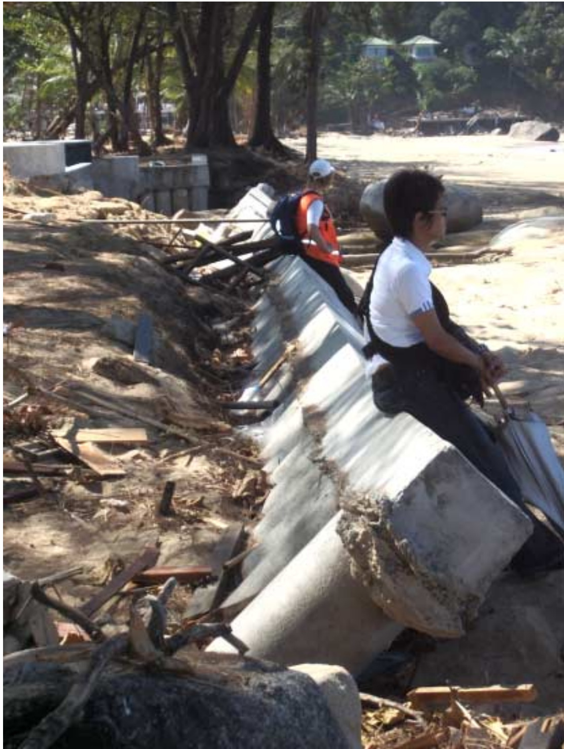
Figure 18. Receding waters (out-rush) caused collapse of most seawall defences from behind due to scouring (Photo RB).
