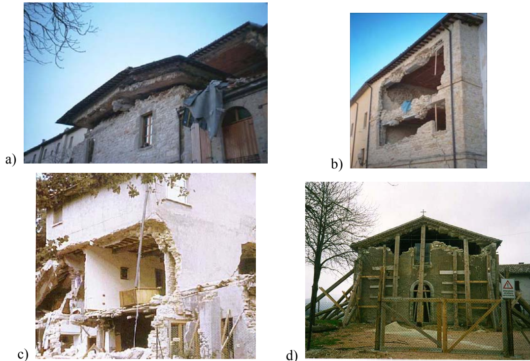
Figure 1. Damages on masonry buildings observed during the Umbria-Marche (Italy) earthquake in 1997. a) b) c) Buildings in Sellano's (PG) historical centre. d) St. Stefano Church in Nocera Umbra (PG).
