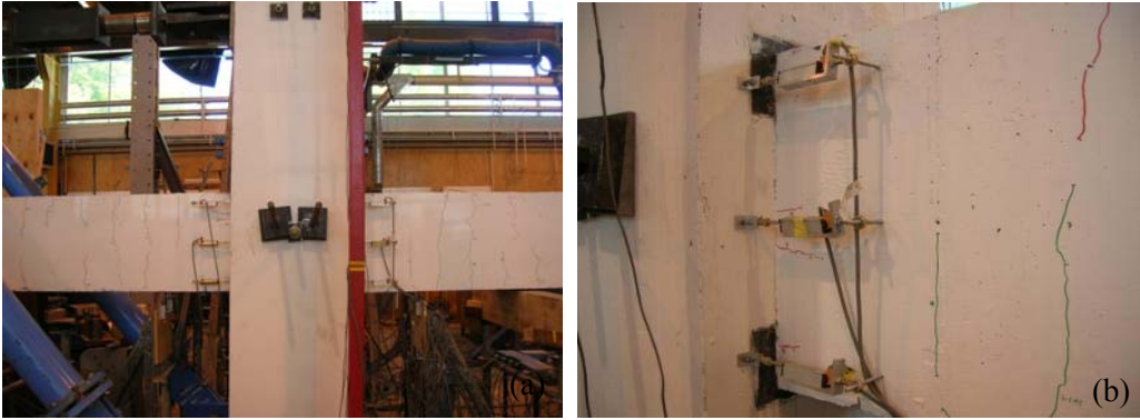
Figure 7: Photographs of the specimen after uni-directional QS testing: (a) the specimen at approximately 3 percent drift; (b) the west beam after completion of testing.
