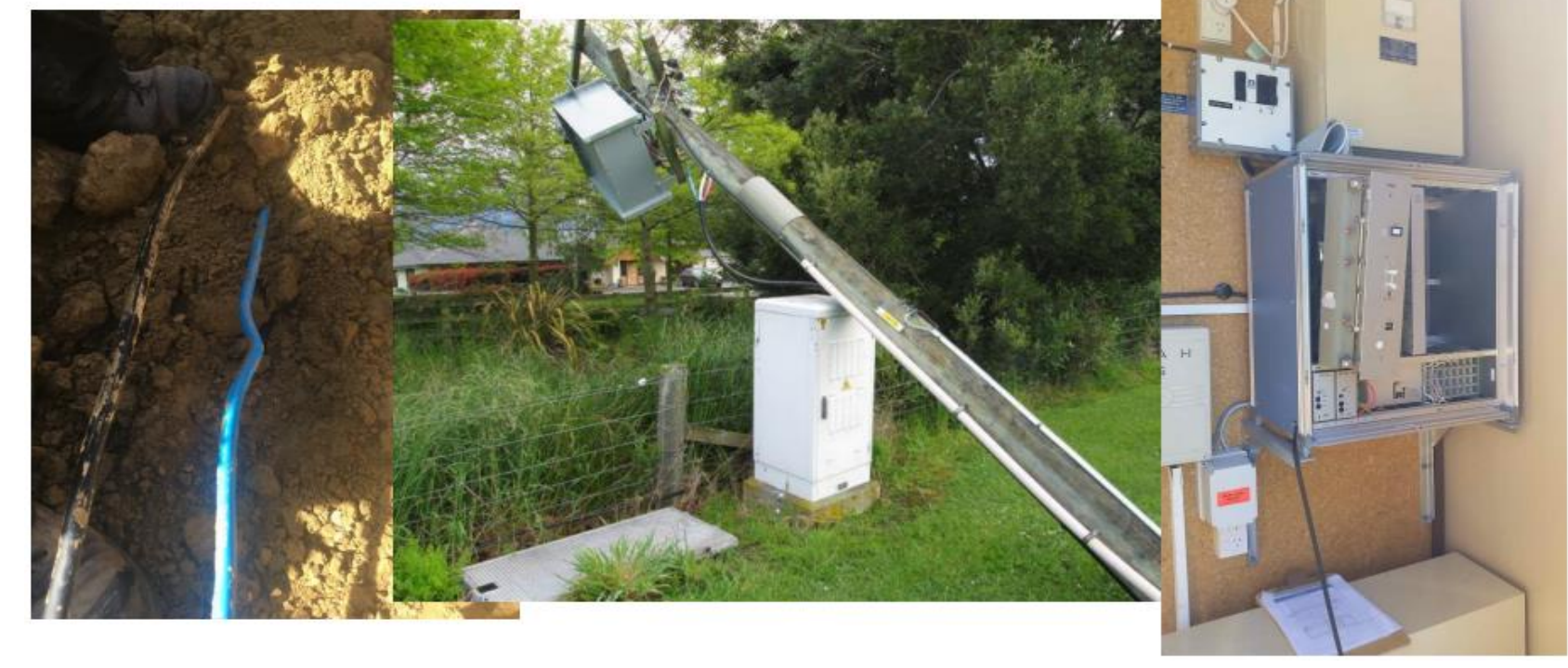
Examples of damage to communications infrastructure following the 2016 Kaikōura earthquake (after Austin 2017)
