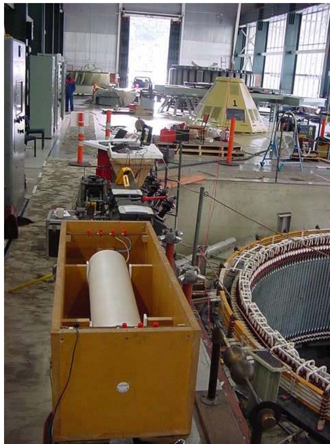
Fig. 2 Resonant inductor in use at Matahina
