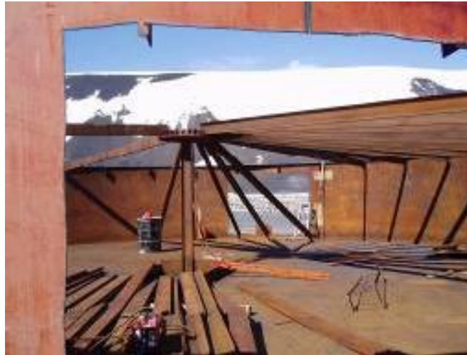
FIGURE 10: THE BULK FUEL TANK DURING THE 6 WEEK REMOVAL. COURTESY OF THE ANTARCTIC TREATY CONSULTATIVE REPORT 2006
