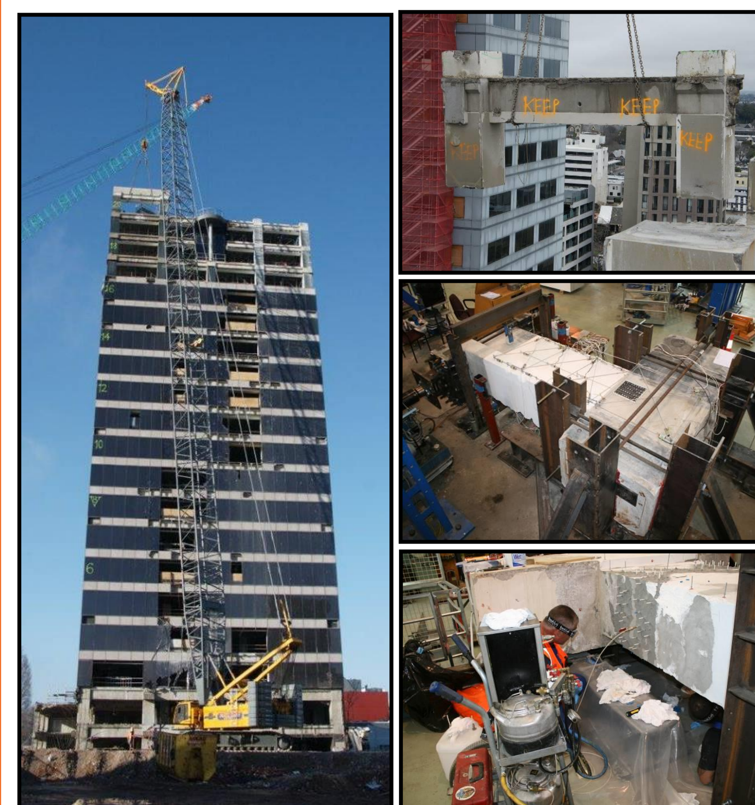
Figure 7: Elevation of the PWC building during the deconstruction process (left); extraction of one of the "H" frames (upper-right); test setup (middle-right); and resin injection of cracks (lower-right).
