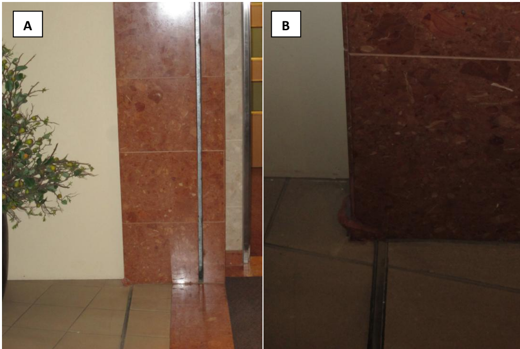
Figure 3.12: (A) Separation Joint in the Canon Wilford wing adjacent to lift shaft. (B) Cosmetic damage to columns adjacent to a vertically displaced separation joint
