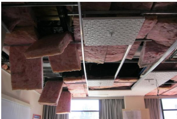
Figure 3.6: Damage to nonstructural ceiling tiles in Christchurch Hospital.
