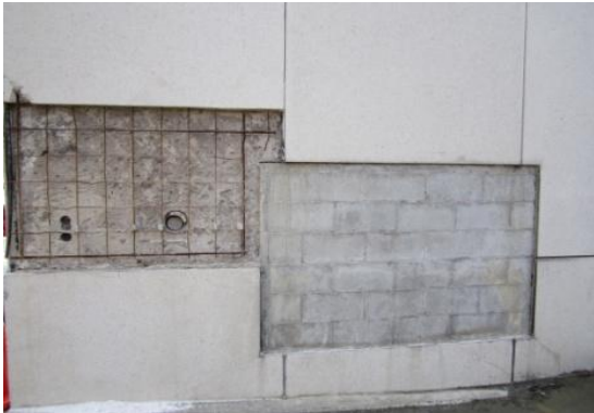
Figure 3.5: Damaged shear wall panels Riverside building, Christchurch Hospital.
