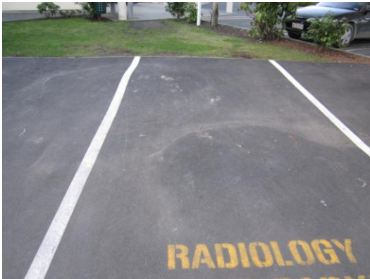
Figure 3.11: Liquefaction induced blistering in the Radiology car park
