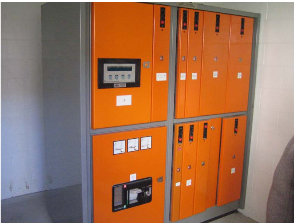
Figure A2.3: Low voltage switchgear
