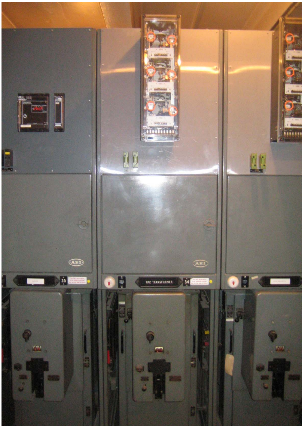
Figure A1.4: High voltage switchgear
