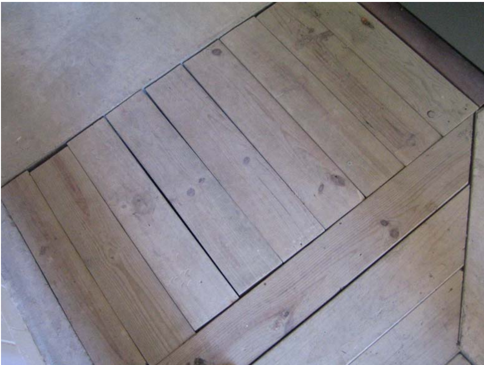
Figure A2.5: Combustible material (wooden board) in a distribution substation
