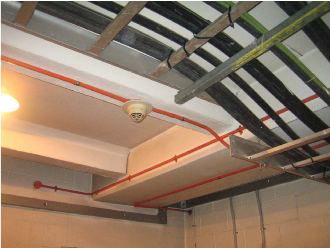
Figure A1.6: Cable tray
