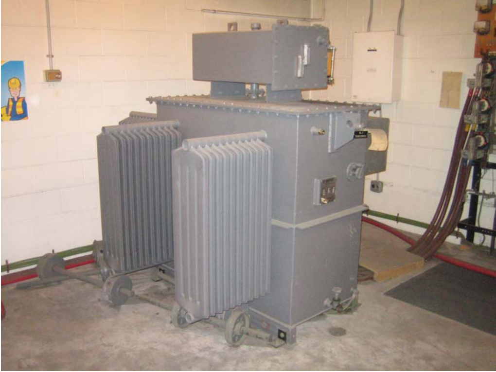
Figure A1.1: 750kVA mineral oil fluid transformer
