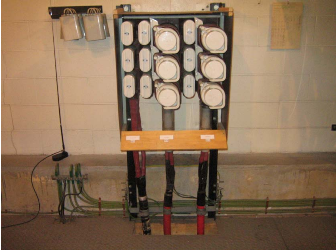
Figure A1.5: Low voltage switchgear
