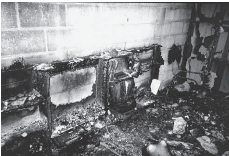
Total loss of family heirlooms in a post-flashover house fire
