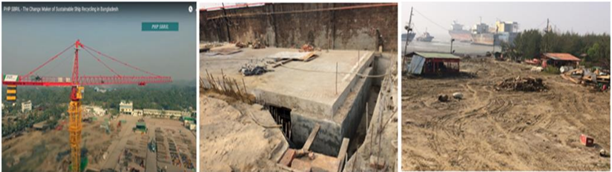
Figure 4.1 Photographic evidence of High, Medium & Low level of Yard Floor
