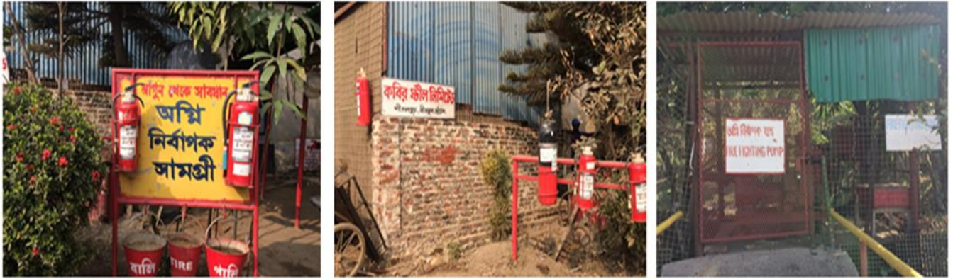
Figure 4.11 Photographic evidence of High, Medium & Low level of Firefighting Facilities
