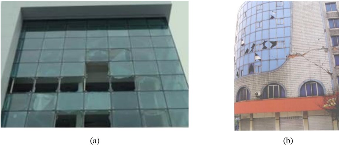
Fig. 1 – Glazed curtain wall damage observed in past earthquakes: (a) 2011 Christchurch Earthquake [1], (b) 2008 Wenchuan Earthquake [2].
