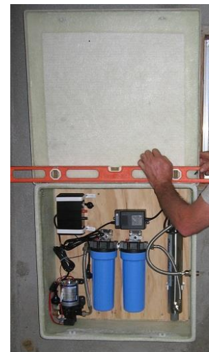
Figure 5.7 Safe water station consisting of a pump, coarse and fine filters, UV-irradiator, 240/12V inverter and 12V cable attachment points.
