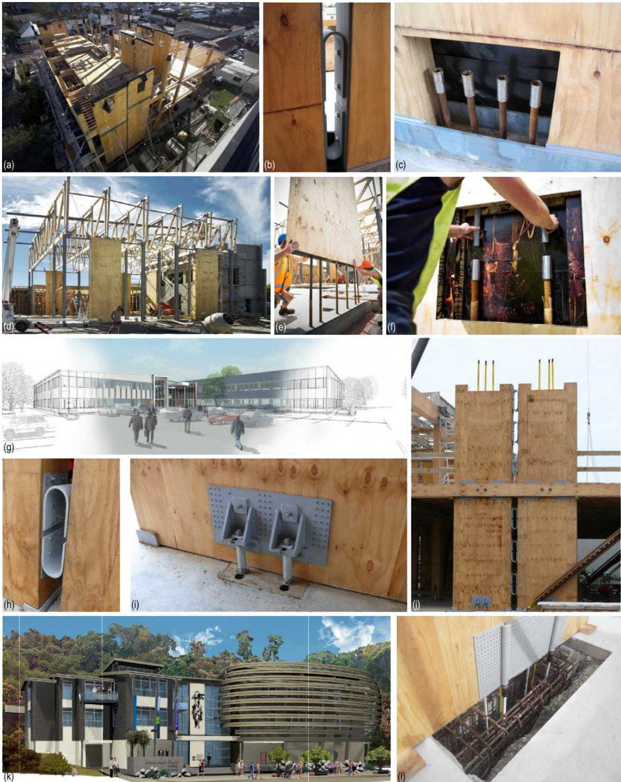
Figure 2. Nelson and Marlborough Institute of Technology (Nelson) (Devereux et al., 2011): (a) aerial view of the construction site; (b) UFP and (c) post-tensioning couplers detail. Carterton Events Centre (Carterton) (Palermo et al., 2012): (d) view of the building under construction; (e) wall base detail under erection; (f) post-tensioning coupling. Trimble building (Christchurch): (g) architectural render (Brown et al., 2012); (h) UFP and (i) base dissipater details; (j) view of the coupled walls (c/o D. Moroder) . Kaikoura District Council Building: (k) architectural render; (l) detail of the dissipaters base connection (c/o A. Buchanan).
