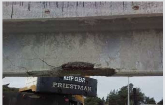
Typical cracking pattern emanating from corroded area
