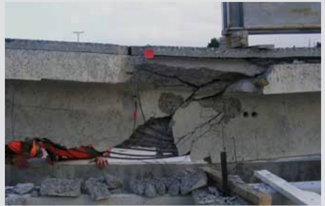
Corroded strands failed and pulled through to separate failure crack at loading point
