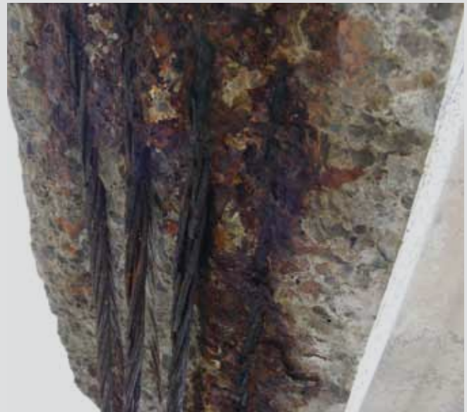
Evidence of upward strand corrosion
