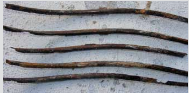
Individual wires with pitting damage
