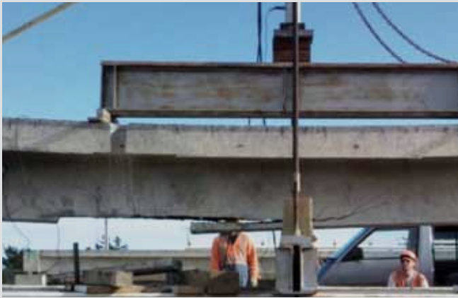
Delamination of soffit in corroded region
