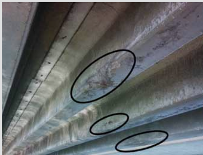
Corrosion-induced cracking in three beams from one span
