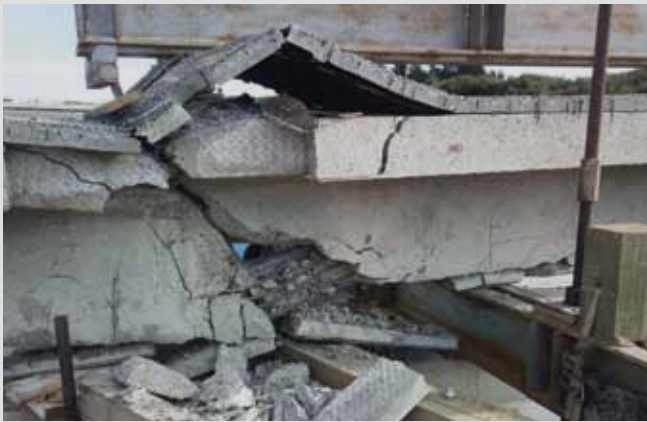
Failure crack location emanating from corroded area to loading point
