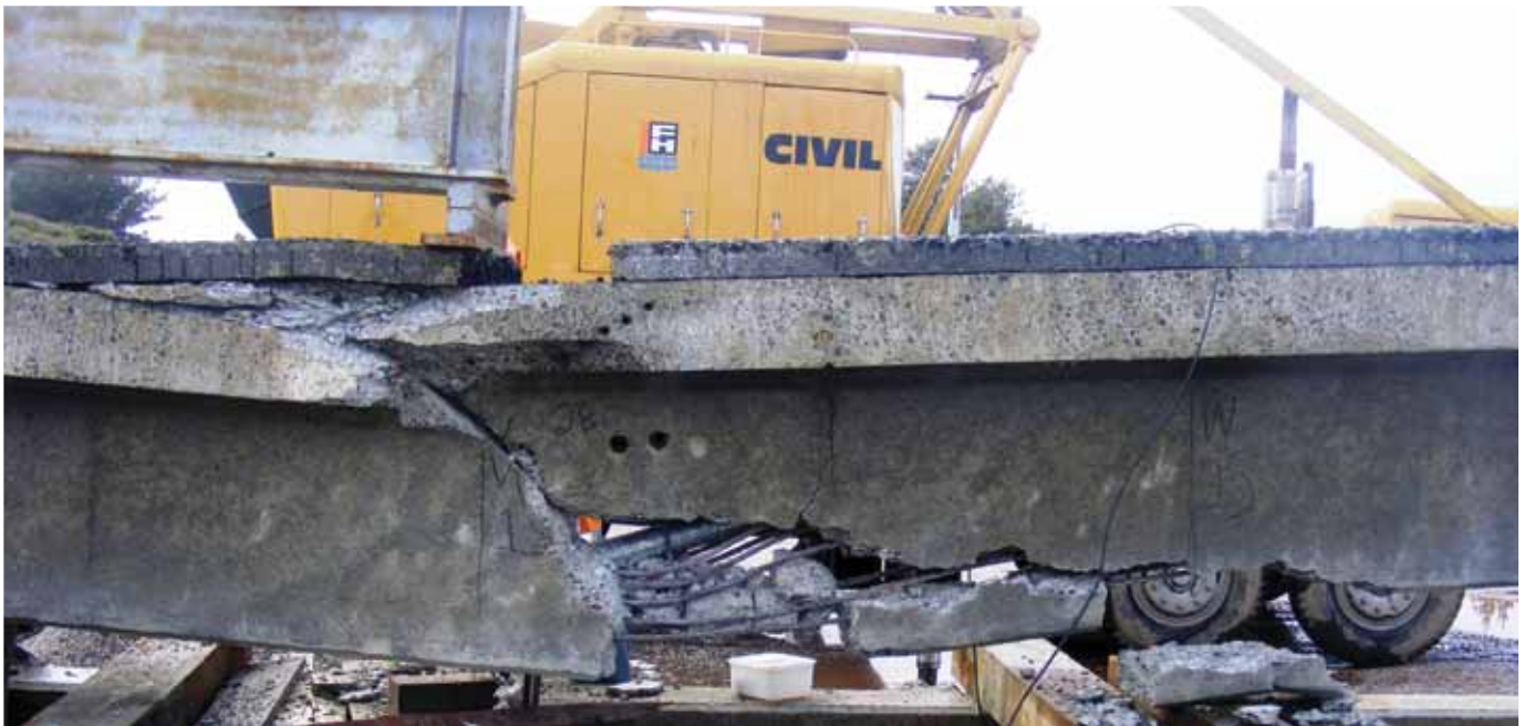
Figure 12. Typical good-condition failure crack.
