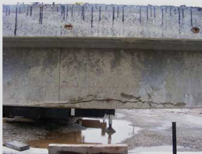
Close-up of corrosion crack in one beam
