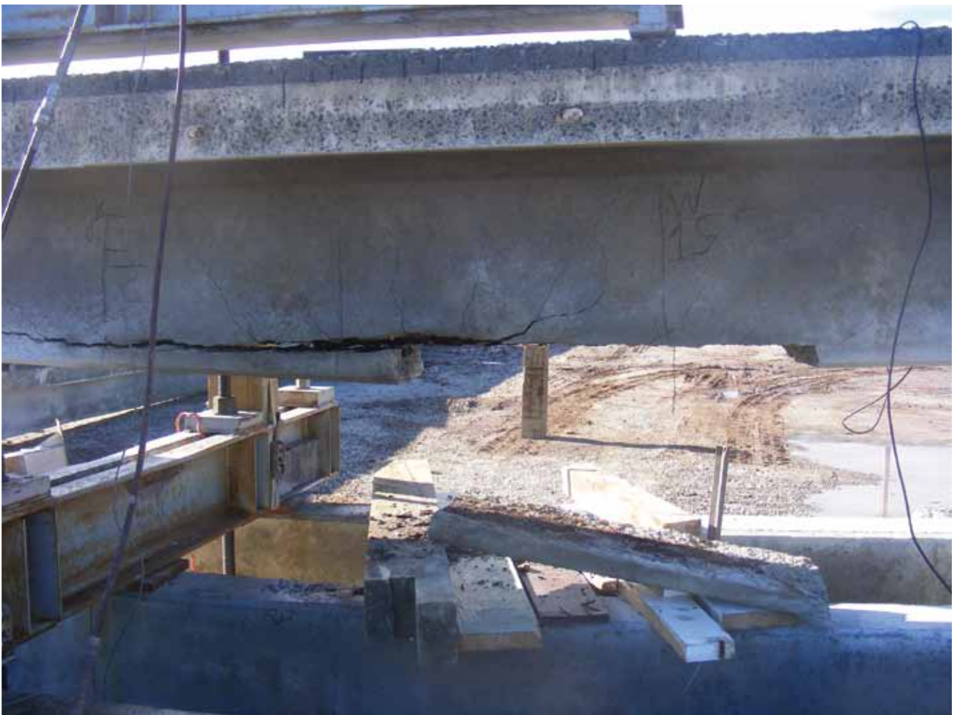
Figure 9. Evidence of soffit delamination during a destructive test.
