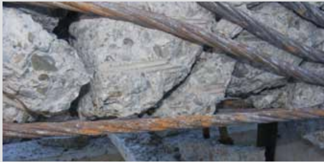
Broken-out strands with uniform corrosion
