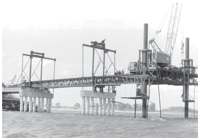
Figure 2. Tiwai Point Bridge launcher in operation in 1967. Photo courtesy of Ray Price.
