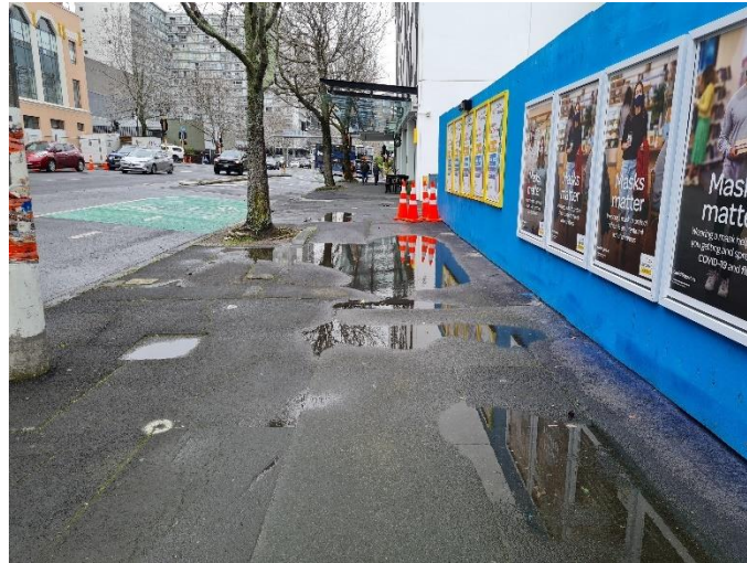
Figure 6. An uneven surface that has cumulated water.
