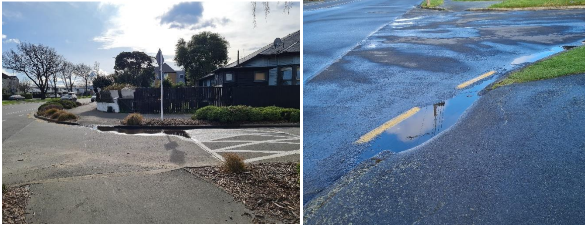
Figure 17. Examples of kerb cut blocked by water days after a heavy rain.
