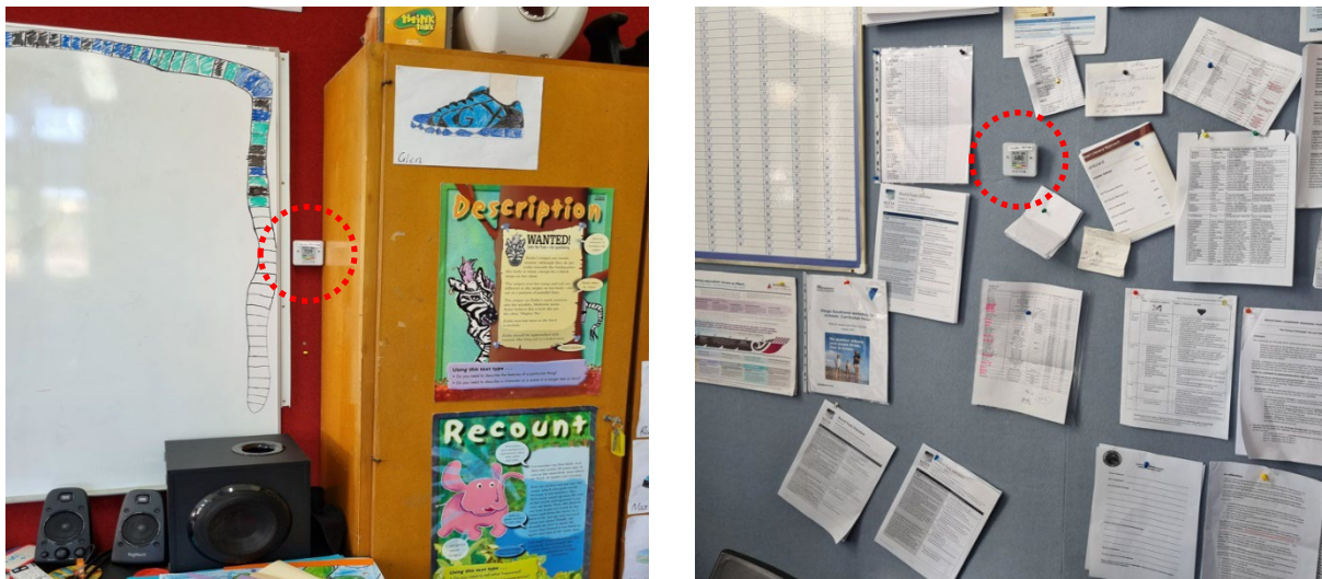
Figure 4: Aranet4 PRO monitors installed on the classroom walls.
