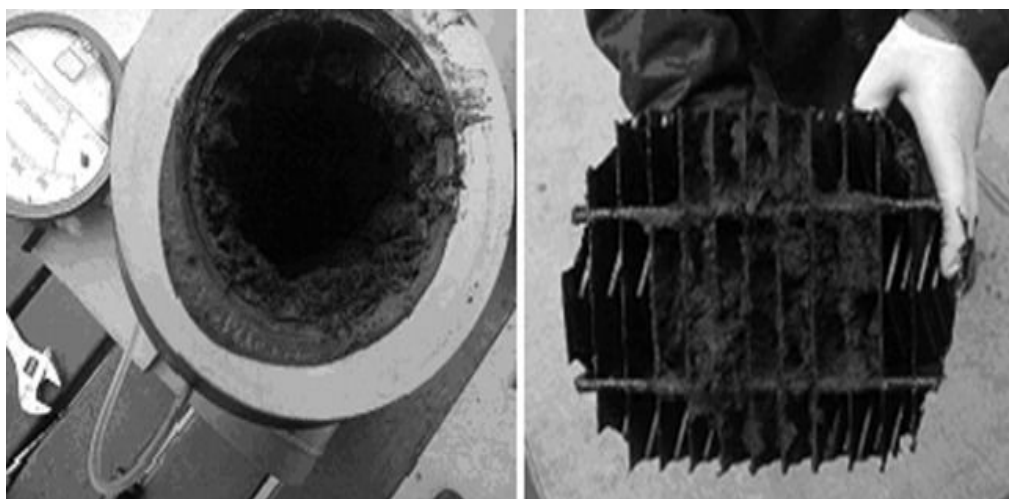
Figure 2.3: Plugging of piping and fouling of equipment (Zwart et al., 2009)
