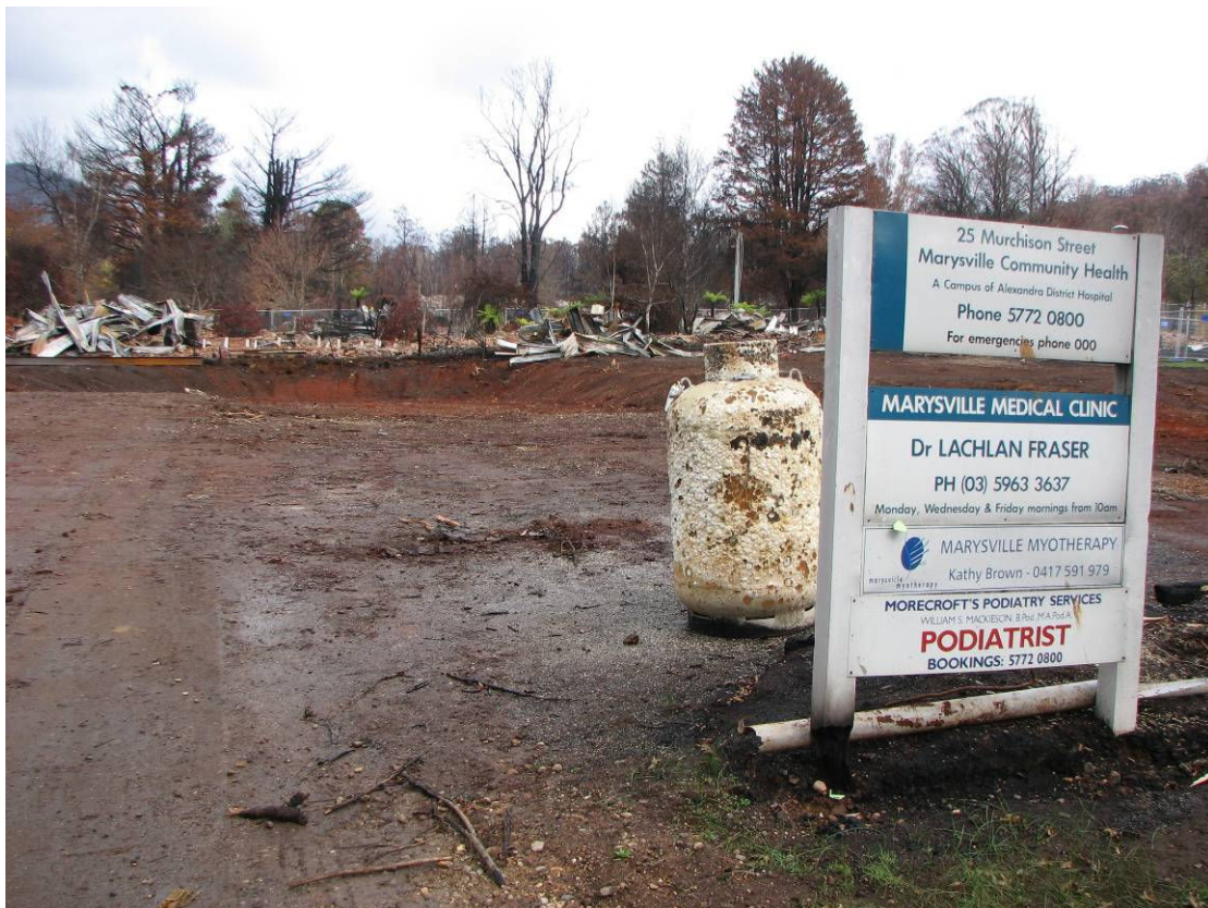
Figure 5.3 The Marysville Medical Clinic after demolition and debris removal (Photo credit: Dr. Lachlan Fraser)
