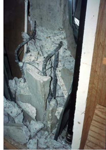
b) Indian Hills Medical Centre, Northridge, 1994
