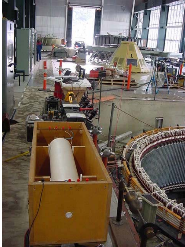
Fig. 1 Resonant inductor in use at Matahina
