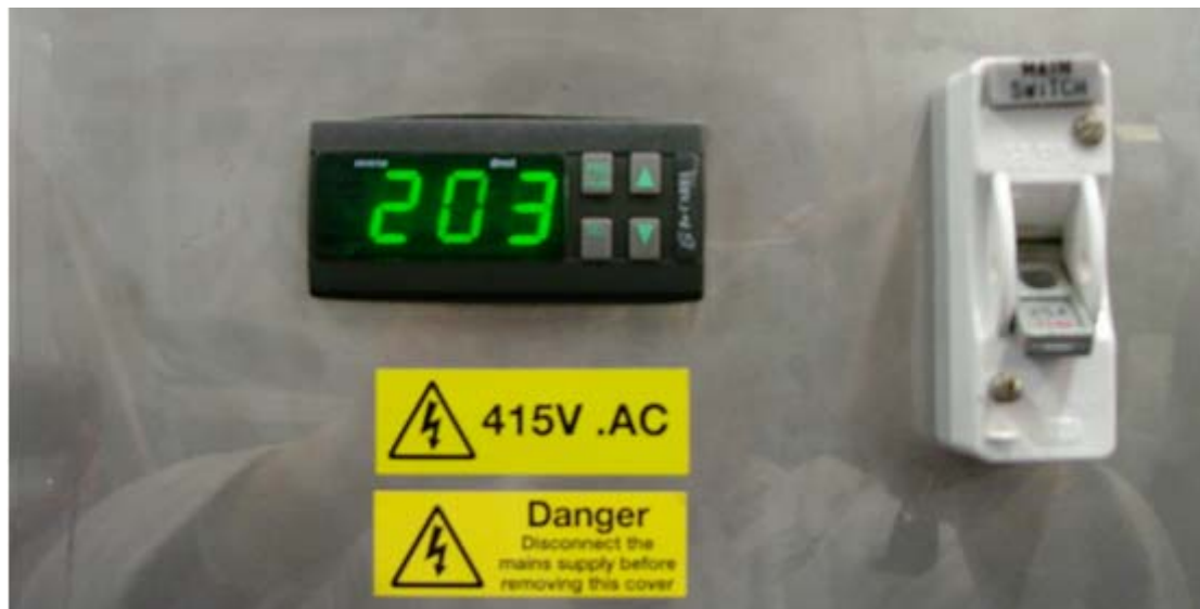
Figure 3.9: Temperature control panel
