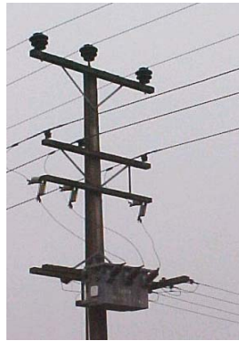
Figure 4: 33kV overhead distribution lines above 11kV lines with Tee-off to local service 11kV/415V transformer
