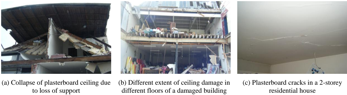
Figure 3: Typical damage to residential plasterboard ceilings.
