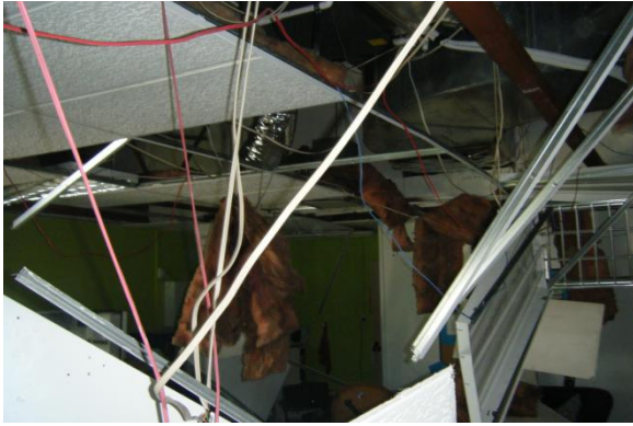
Failure of splice connection of the main beam
