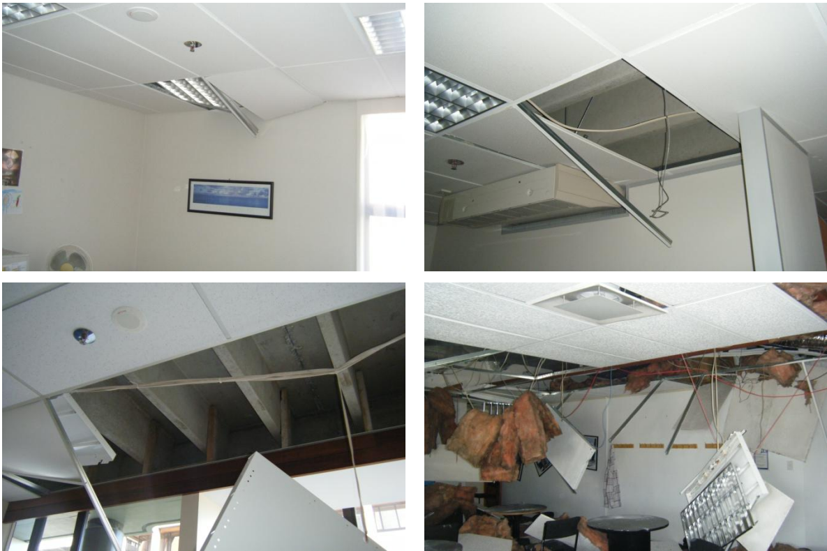
Figure 6: Localised ceiling damage due to failure of the grid members to wall angle connection.
