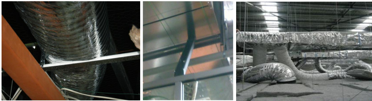
HVAC pipe supported by ceiling grid Glazed wall braced to AC unit Unbraced AC ducts resting on the ceiling
