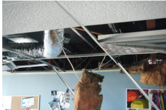
Damage to a large (7m x 12m) ceiling
