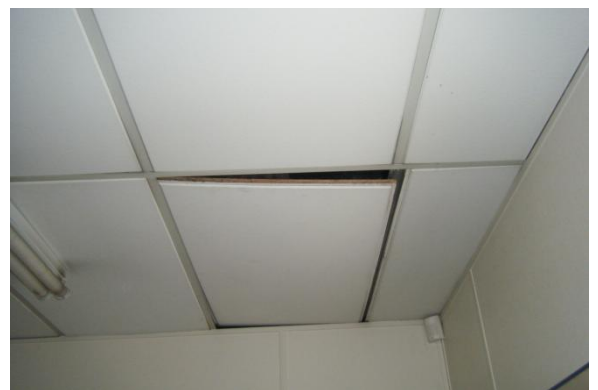
Damage to flange of the grid beam due to tile impact
