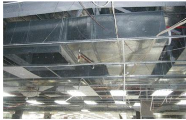
Damaged ceiling with inadequate service height
