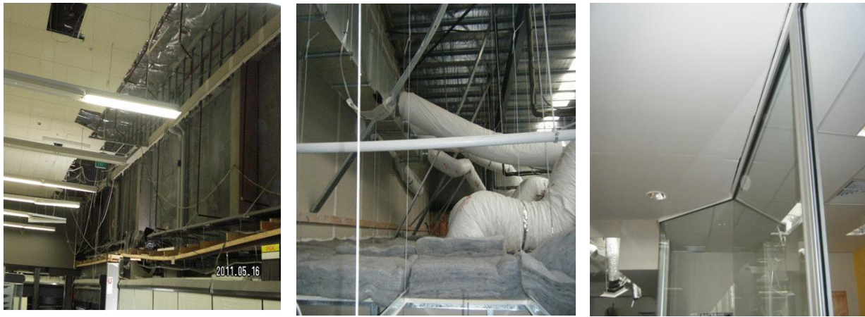
Damage to ceiling and bulkhead
