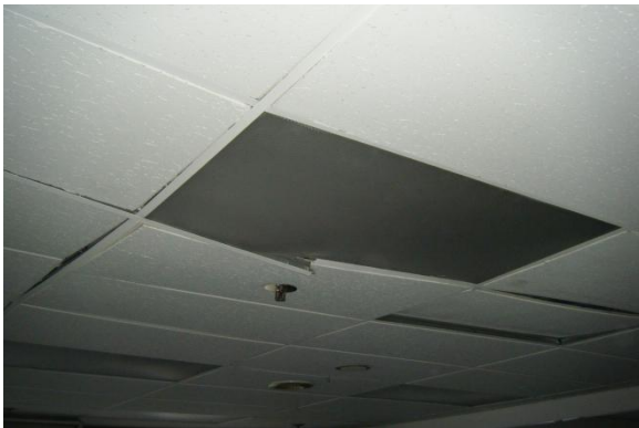
Localised damage to ceiling grid and tile due to interaction with sprinkler
