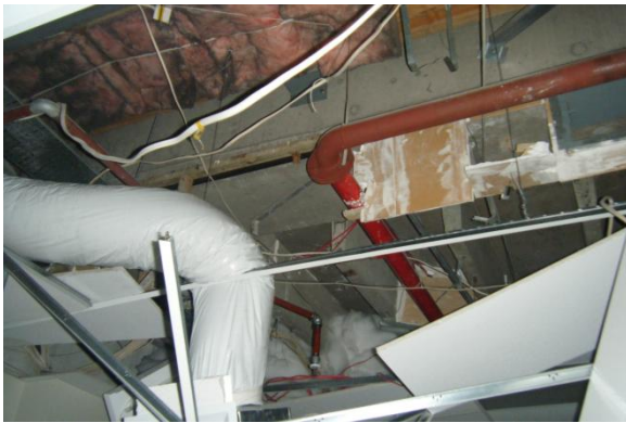
Ceiling damage in the upper floor with heavy tiles
