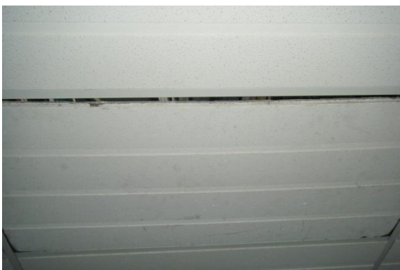
Dislocation of ceiling tile due to vertical acceleration
