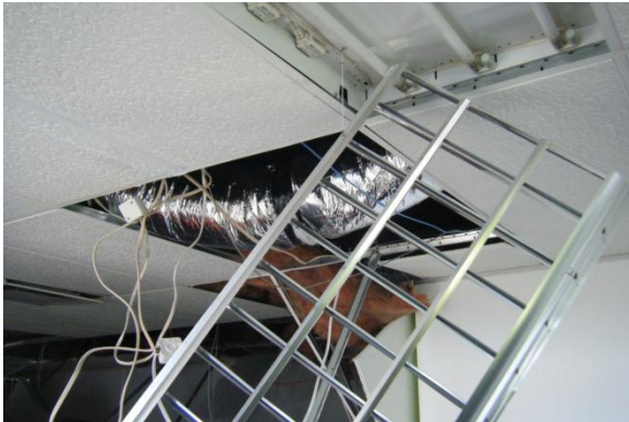
Damage incurred to a small ceiling
