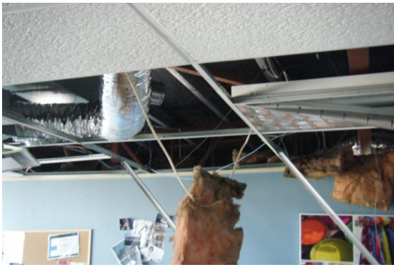
Ceiling damage caused by unbraced AC ducts
