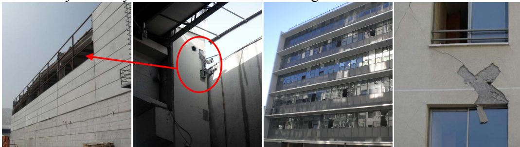
Figure 1: Example of cladding failures
