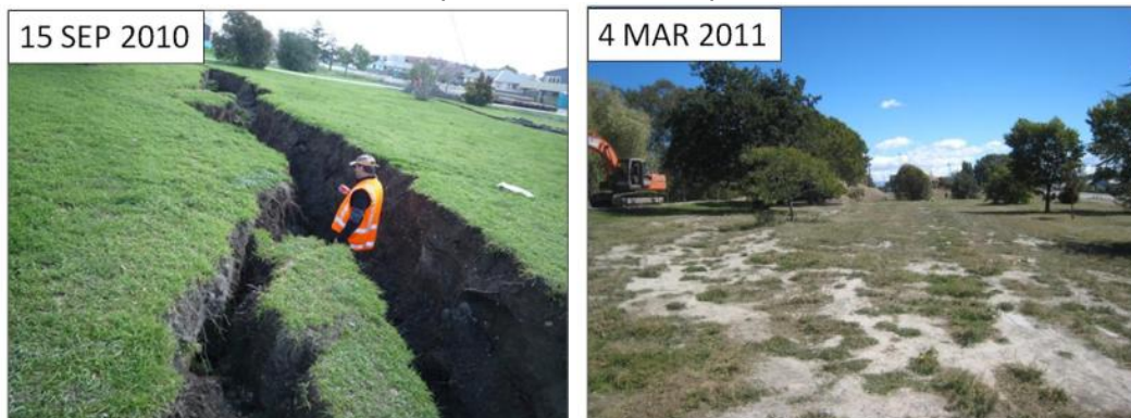
Figure 21. Damage to the stop bank along Kaiapoi river (North Kaiapoi). Sand boils were observed on restored cracks. The damage to the stop bank was minor and lots of small fissures were observed at restored cracks.
