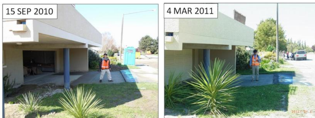
Figure 22. Further subsidence in two-story house neighboring the stop bank. (North Kaiapoi)
