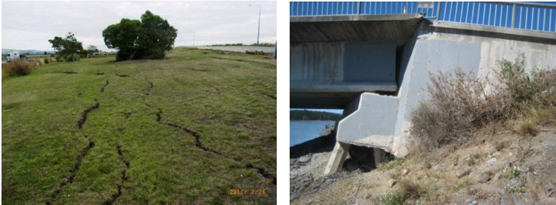
Figure 18. Liquefaction-induced damage to South Brighton Bridge.
