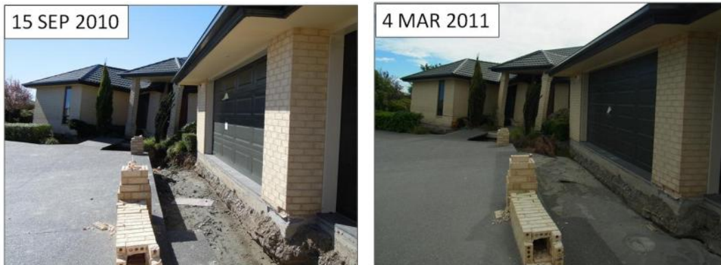
Figure 19. Minor additional damage to a residential house which underwent foundation failure due to lateral spreading and liquefaction in 2010 Darfield Earthquake. (South Kaiapoi)
