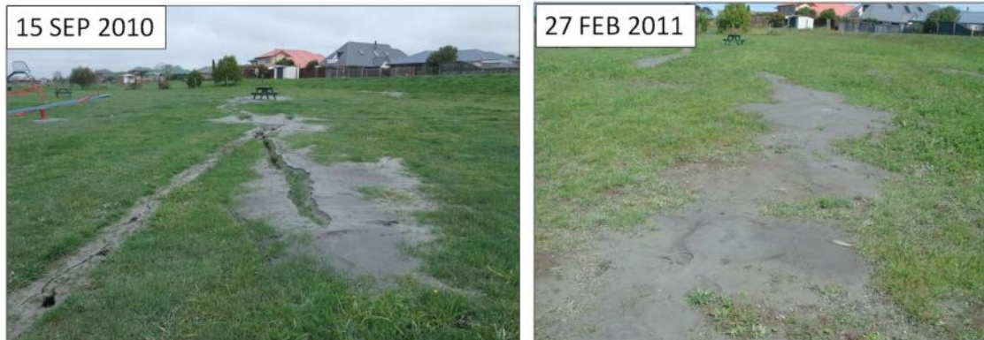
Figure 20. Repeated liquefaction at a park adjacent to Courtenay Lake (South Kaiapoi). Liquefied soil was ejected from existing cracks, but ground distortion was minor compared to the ones observed in September 2010 earthquake.
