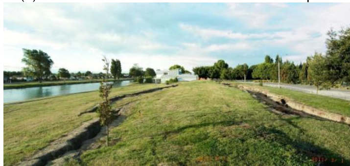
Figure 13. Lateral spreading and the crown settlement of a stop bank near Porritt Park.
