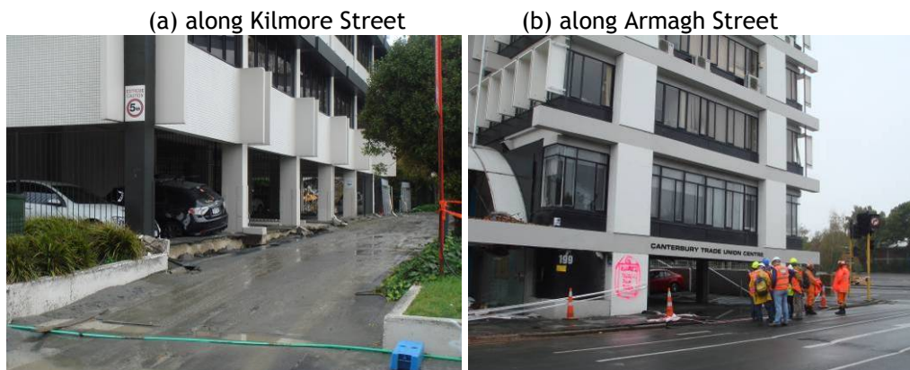
Figure 11. Liquefaction-induced damages in CBD.
