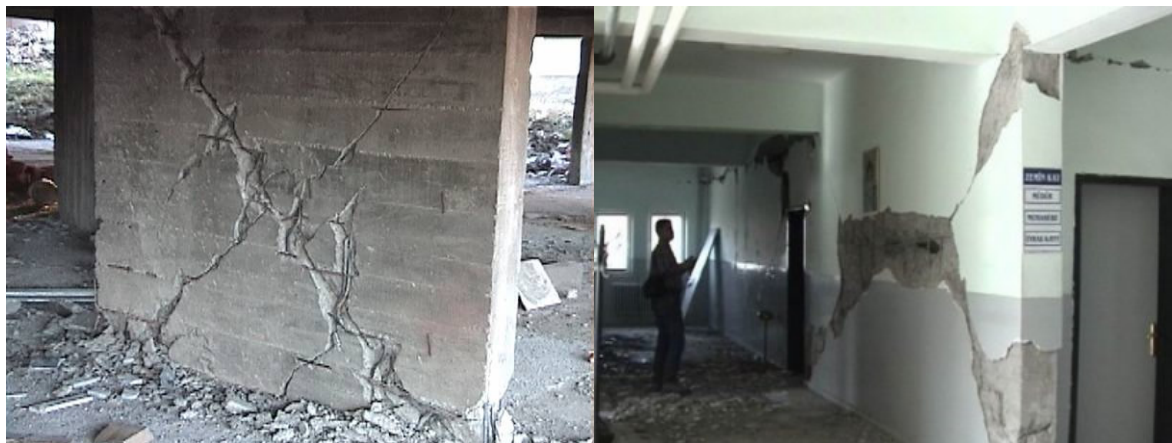
Figure 1: Shear failure of a R.C. due to insufficient transverse reinforcement; a) Bolu (Turkey 1999), b) Bingol (Turkey 2003).
